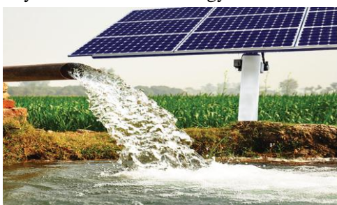
Figure 10 Solar Water Pump System
