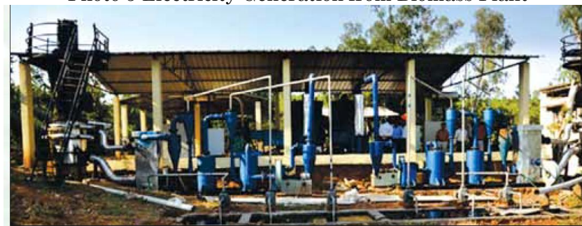
Biomass based decentralized electricity generation system at village Mana, Raisen District
